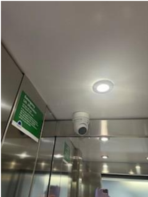
Pic.3. Photo of CCTV Camera in Lift H114 (Block A)
